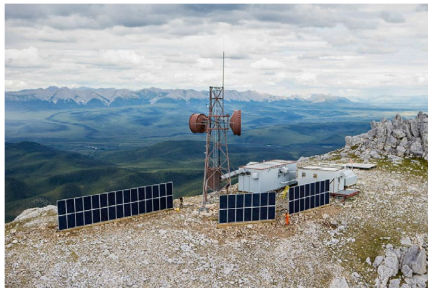
Photovoltaic array on the top of a mountain in the Yukon at Northwestel's Engineer Creek site off the Dempster Highway.
