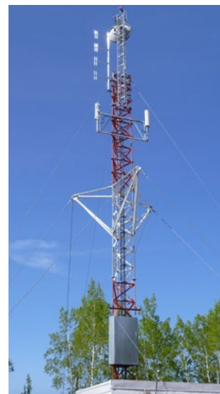
A 4G cell service tower in Wrigley installed in 2014.
